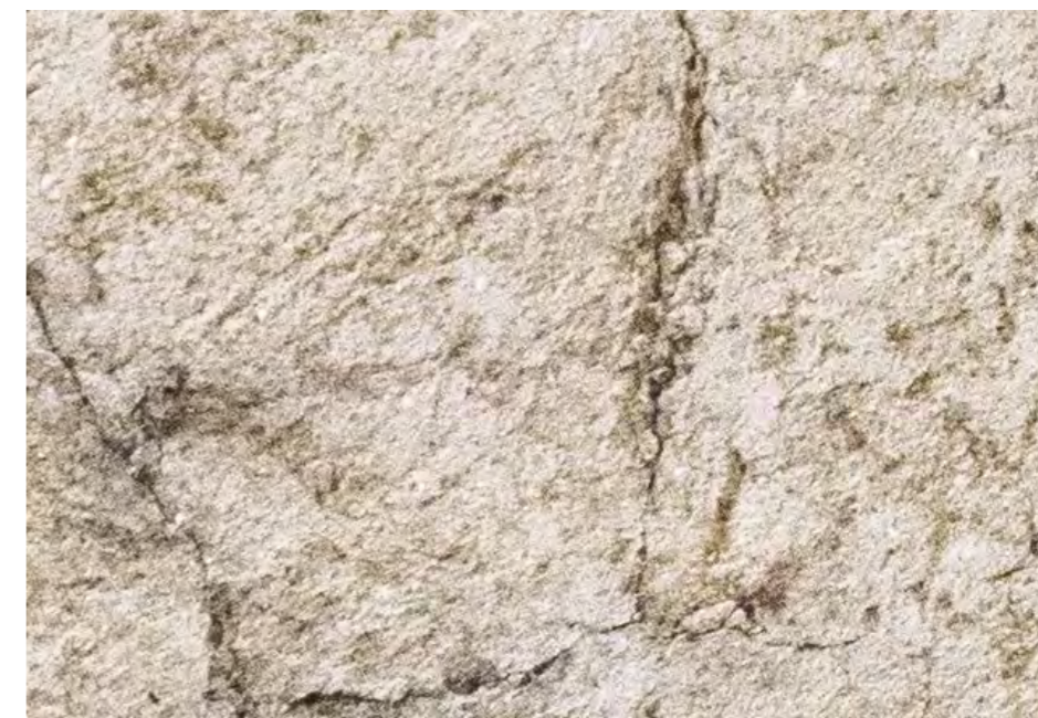
Shrinkage cracks appearing in base coats
