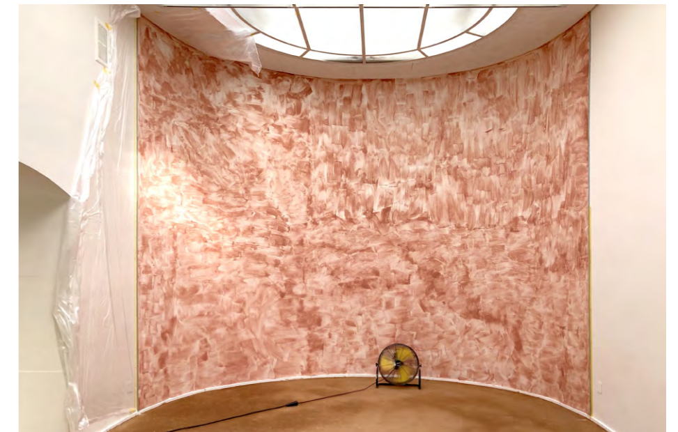
An existing gypsum substrate prepared with structured primer to allow the Léém Clay Plaster to properly anchor on the wall
