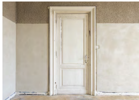
A distance of 5cm is kept between the floor and the Léém Clay Plaster
